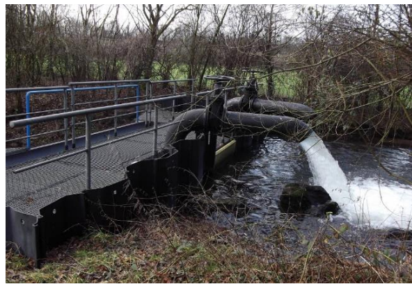
Pumpwerk (Foto: LANUV NW)
